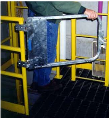
Galvanized Ladder Safety Gate in an Energy Research Facility.
